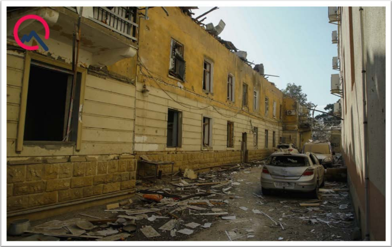
Photo 39: Damage inflicted upon the civilian infrastructure in the city of Ganja
