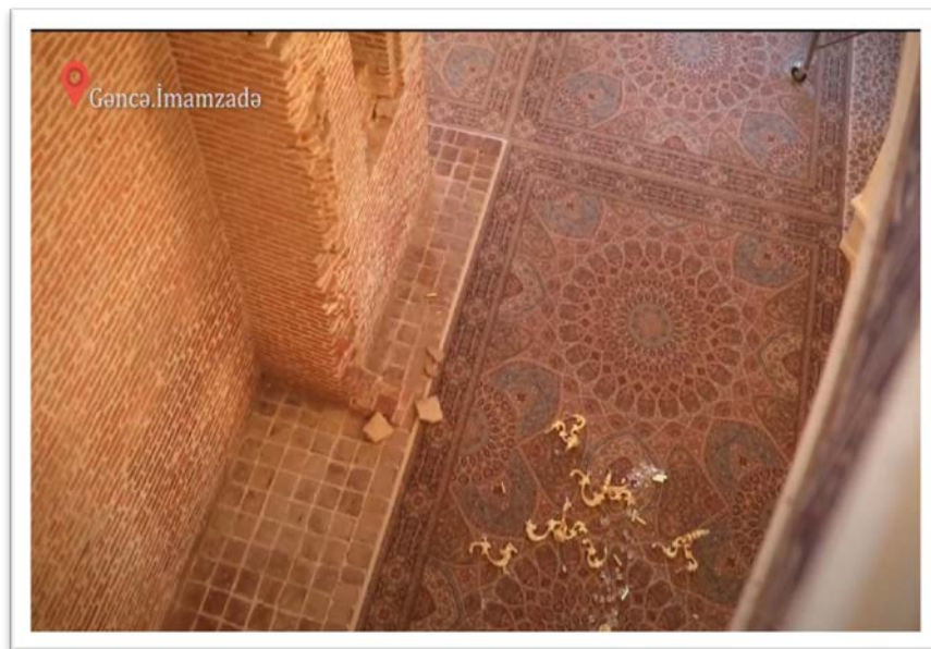
Photo 15: Interior of the Imamzade mosque damaged as a result of the attack on the Ganja city
